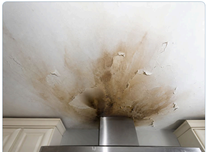
Photo 2 — Ceiling blistering above range
