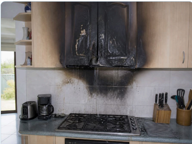
Photo 1 — Cooktop / cabinet heat damage
